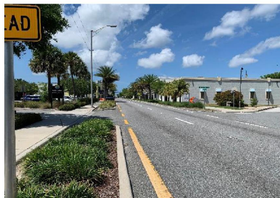
Figure 58 Roadway Surface – South Washington Avenue
