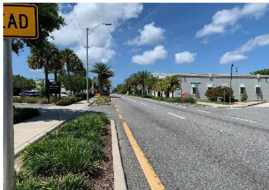
Figure 58 Roadway Surface – South Washington Avenue
