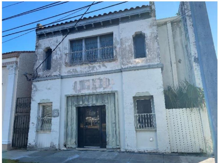
Figure 34. Dilapidated Historic Building
