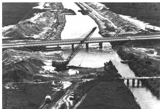
Construction work on the Cross Florida Barge Canal. 1950s. Courtesy of State Archives of Florida, Florida Memory.
